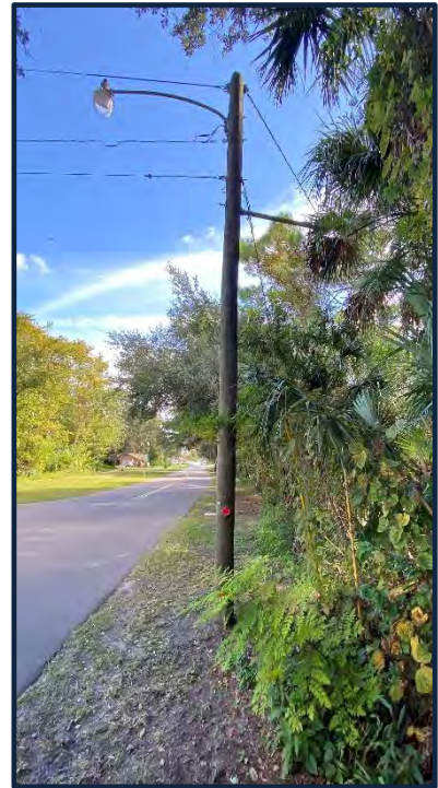
FIGURE 10: ELECTRIC DISTRIBUTION LINES WITH LIGHT FIXTURES ON SOUTH STREET
