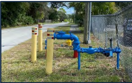
FIGURE 11: FIRE PROTECTION BACKFLOW PREVENTOR ON SOUTH STREET
