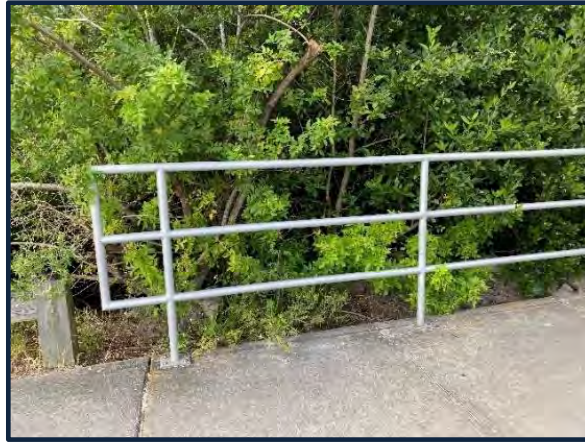
FIGURE 9: EXISTING DAMAGED HEADWALL & CROSS DRAIN #2 AT SUNSET DRIVE
